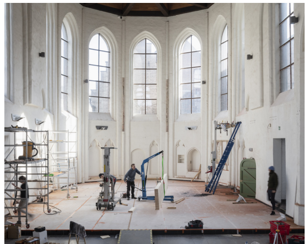
Construction of Spatial Intervention KHG#02 , April 2019. Cinema realised together with Art Cinema OFFoff, design by Olivier Goethals.
