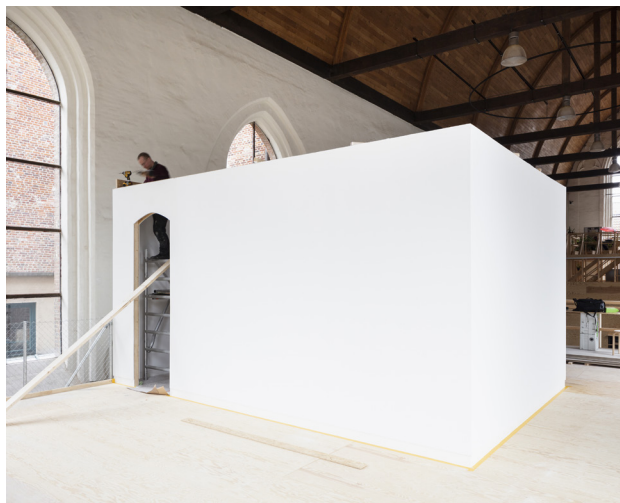
Construction of Spatial Intervention KHG#03 (pavilion and bridge). Design by Olivier Goethals, June 2020.
